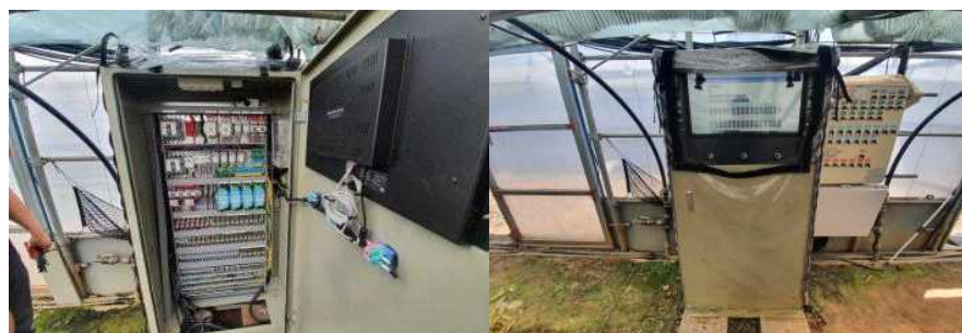
Fig. 20 Heating control system control module
