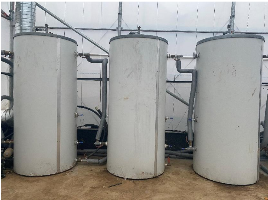
Fig. 11. Hot water storage tank (each tank 1ton).
