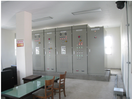
(c) switchboard cubicle
