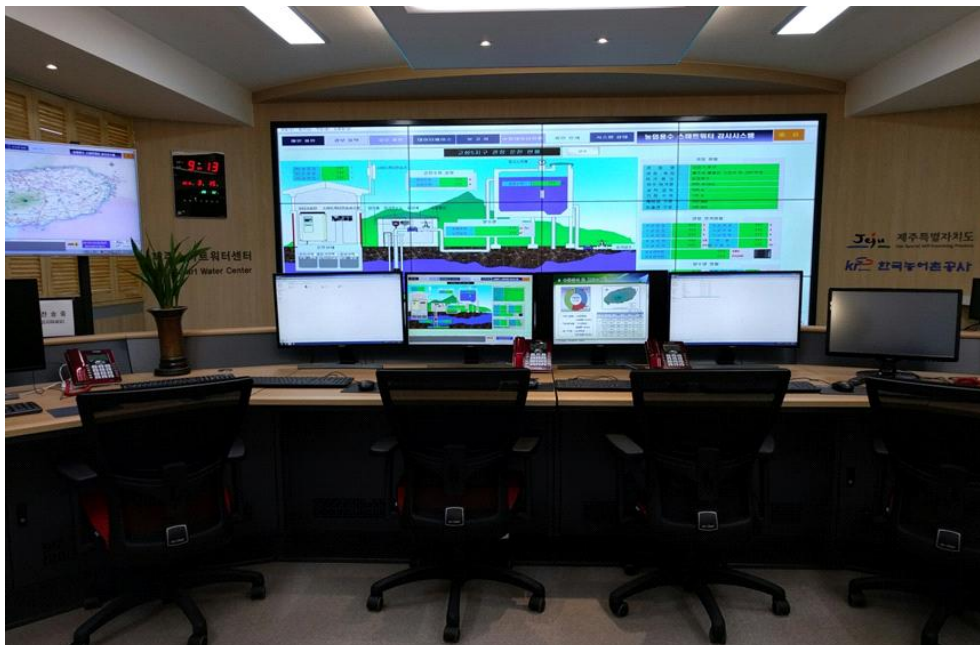
Fig. 5.6 The office of smart-water system in KRC Jeju(한국농어촌공사, 2018)
