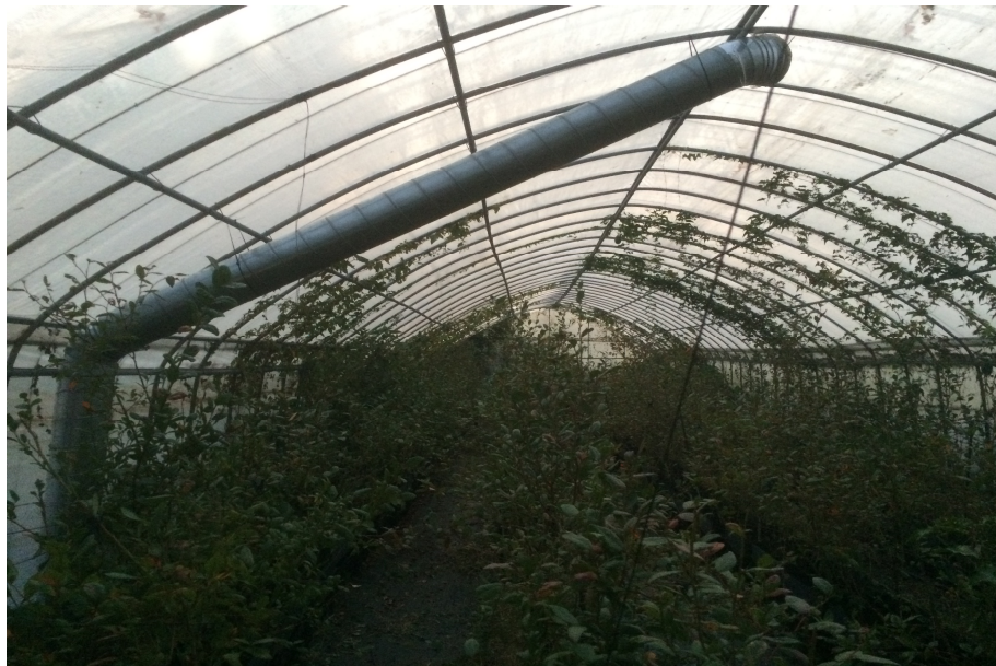
Fig. 10 Picture of the duct in greenhouse
