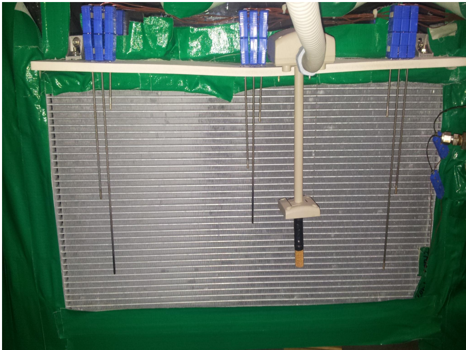
Fig. 13 Condenser of heat pump system
