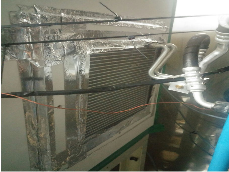
Fig. 12 Evaporator of heat pump system
