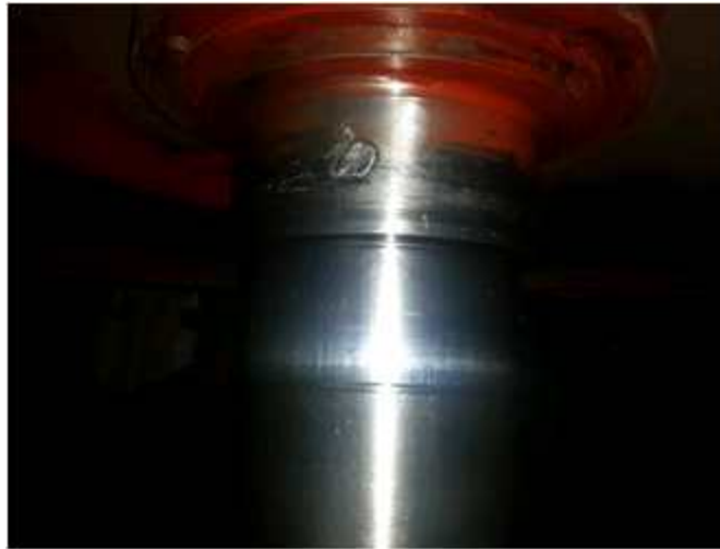
Fig 20. Generator rotor self-welded (Site: 'B' WT of Hankyung wind farm, Date:2014-09-15).
