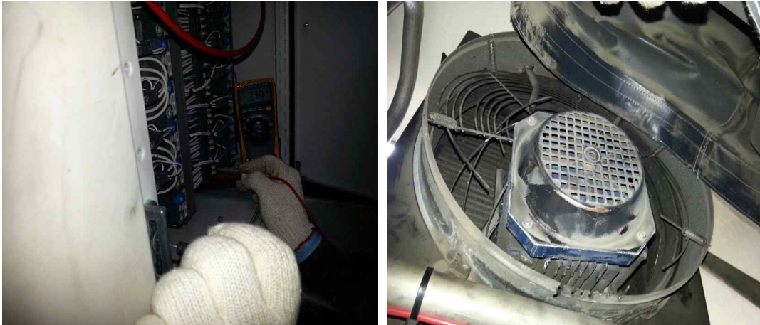
Fig 24. Thermal relay inspection(Left) / Broken nacelle fan(Right).
