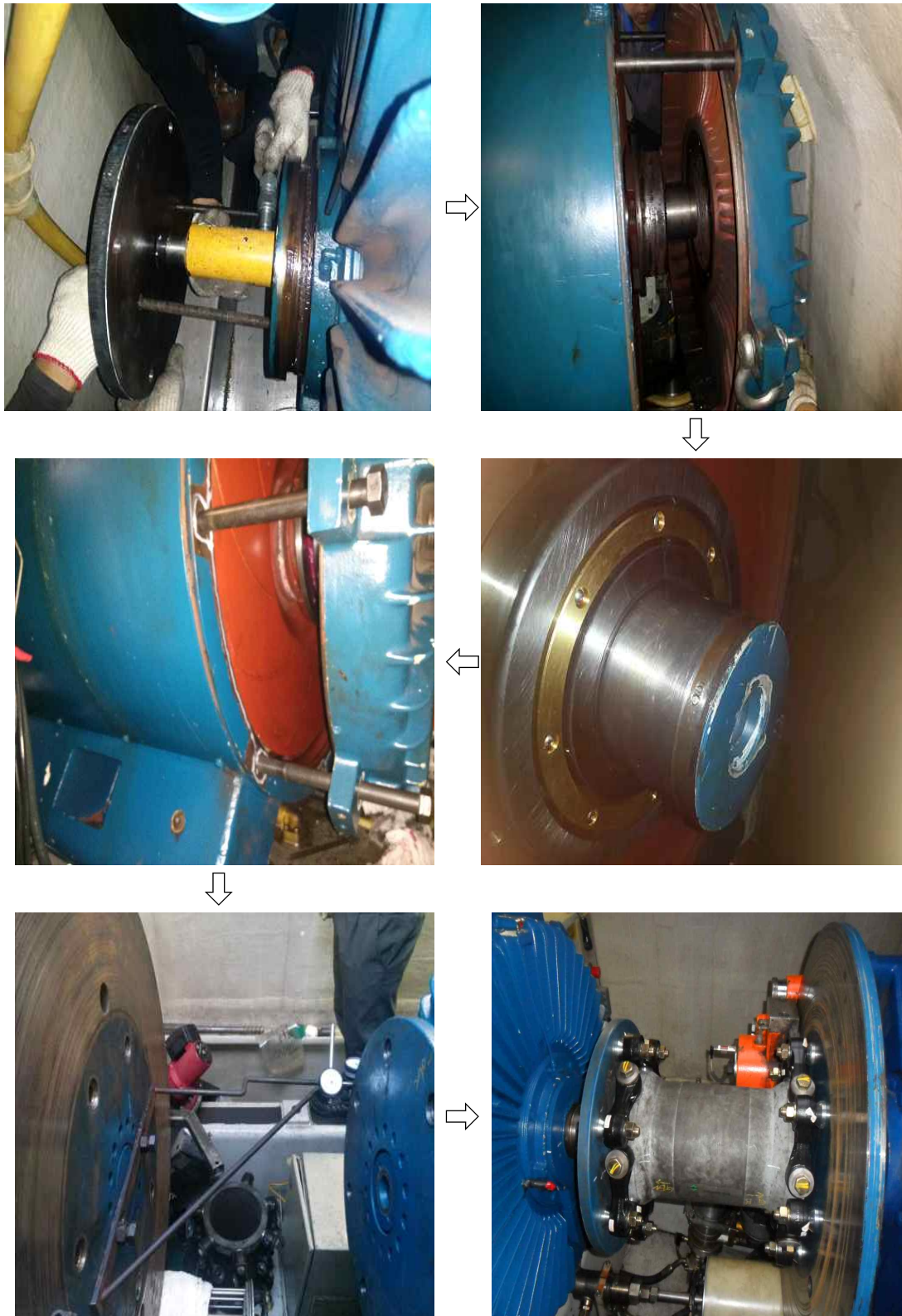
Fig. 21 The process for replacement of the broken generator bearings (Site: 'B' WT of Hankyung wind farm, Date: 2014-09-15~19).
