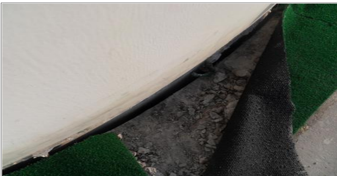
Fig. 17 Foundation damage of No.5 wind turbine at Sungsan wind farm
