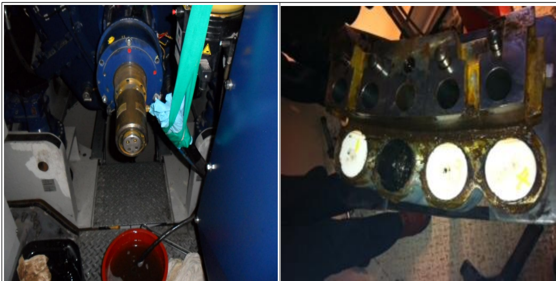
Fig. 21 Rotating unit/yaw claw repair of No. 3 wind turbine at Sungsan wind farm
