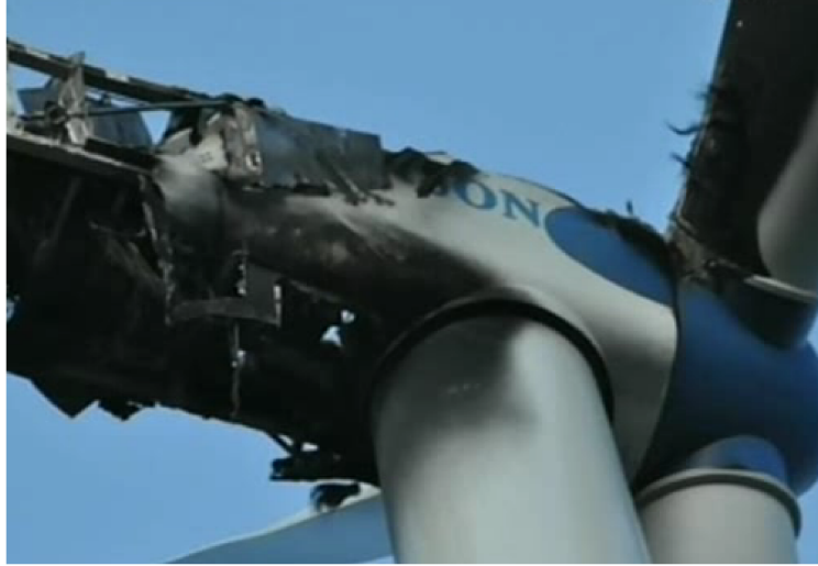
Fig. 3 Yeongheung wind turbine fire
