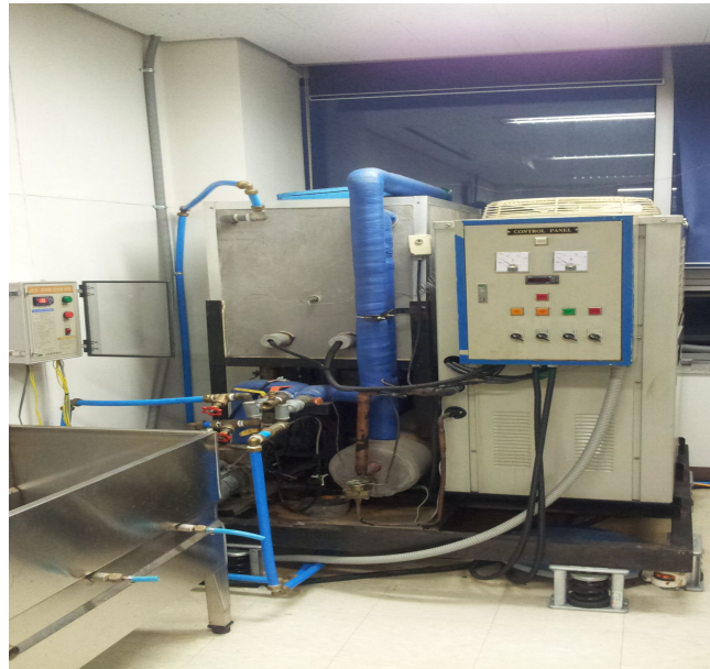
Fig. 8 Photograph of 10.5kW capacity chiller for cooling
