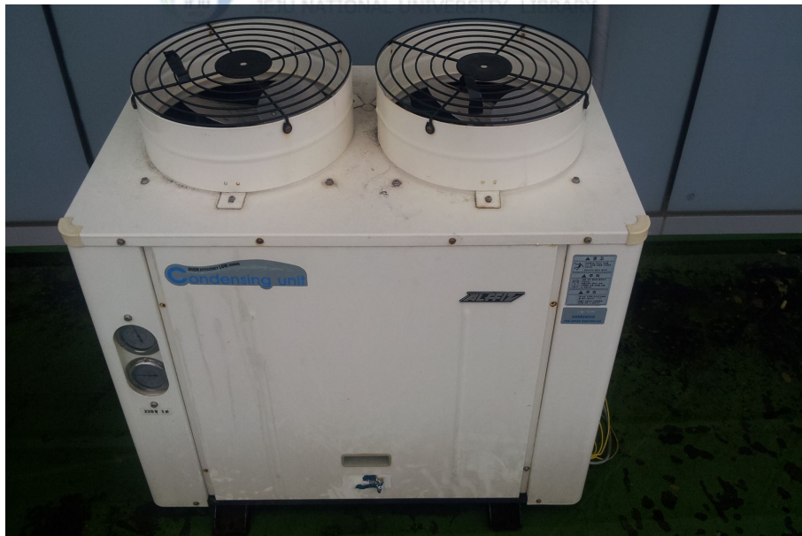
Fig. 9 Photograph of condensing unit
