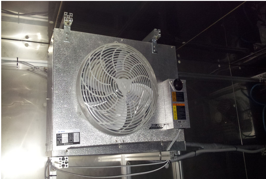
Fig. 10 Photograph of unit cooler
