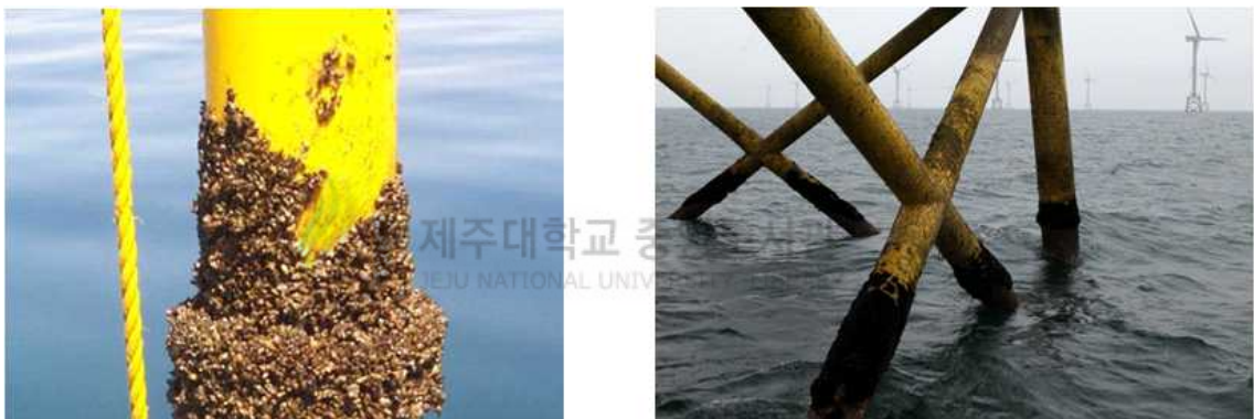
Fig. 4 Marine biofouling on surface of steel members(Jacket)[5]
