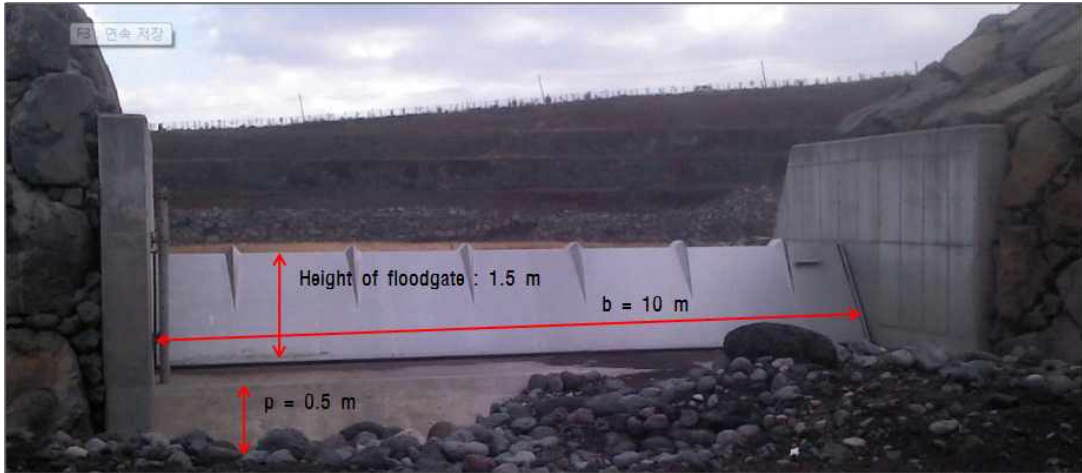
Fig. 4. The front view of the inlet of the first HanCheon Retention pond in HanCheon (Weir).
