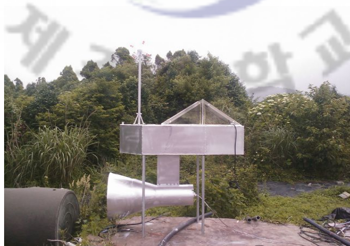
Fig. 28 View of the hybrid generation system
