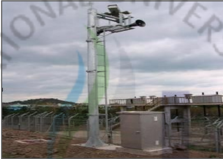
Fig. 4 The installed CCTV camera
