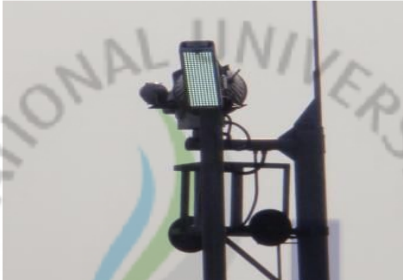
Fig. 13 The arrangement of security equipment
