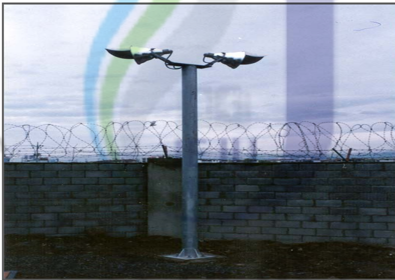
Fig. 5 The installed security lights
