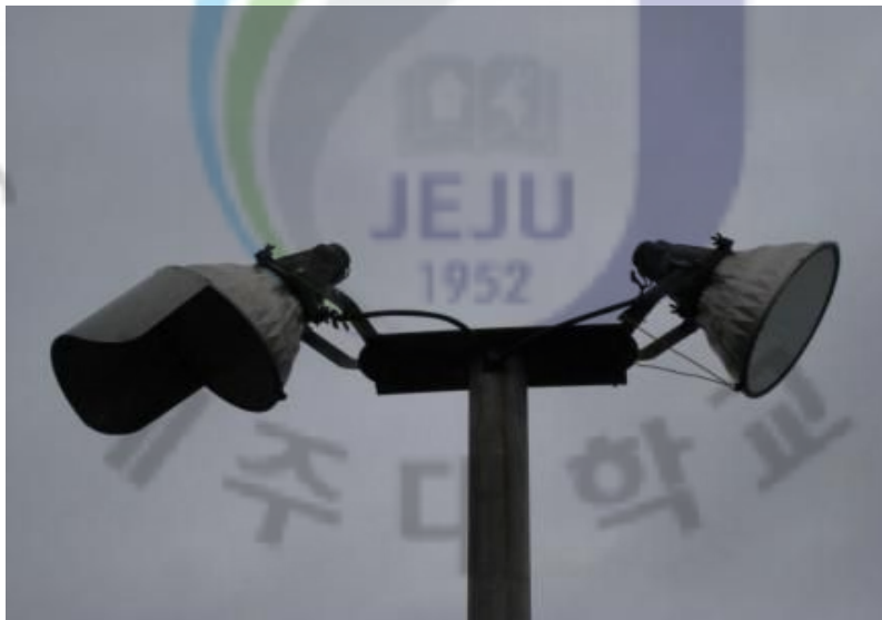
Fig. 9 The installed security luminaire
