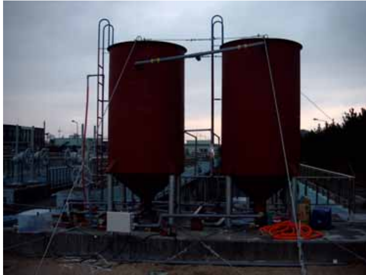
Photo 1. Photo of InSub system for pilot plant
