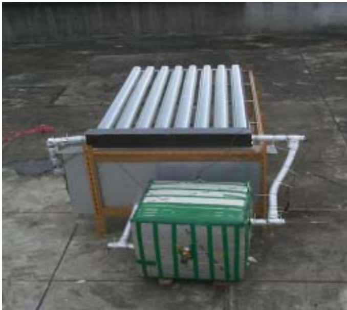
Fig. 18 Photograph of the installed SEIDO 2
