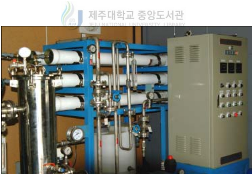
<Picture 4> RO Equipment Built in Pilot Plant
