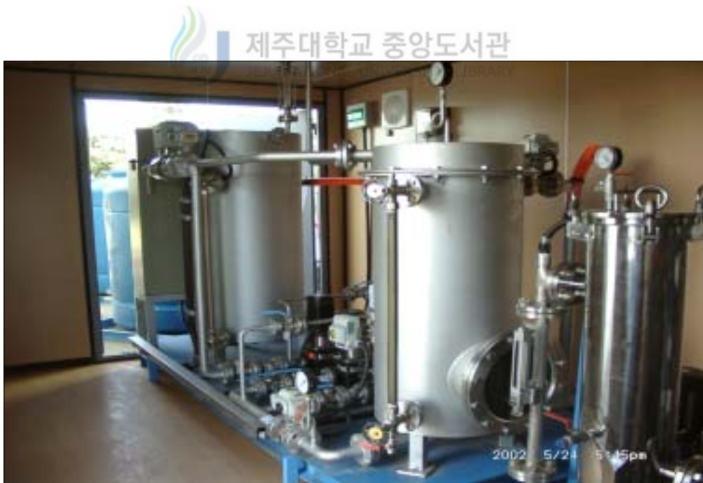
<Picture 3> BMF Equipment Built in Pilot Plant
