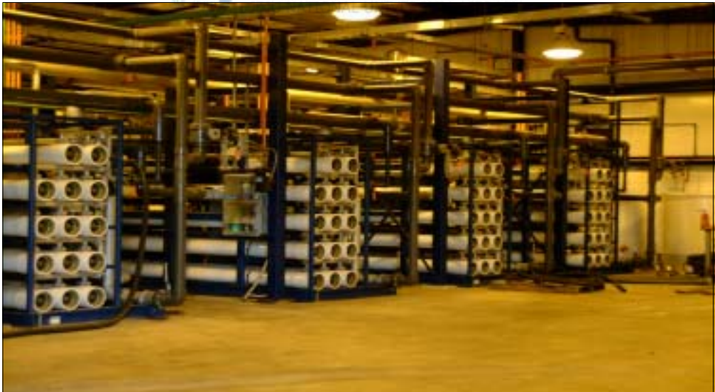
<Picture 1> RO Equipment of Honouliuli Wastewater Treatment Facility in Ohau, Hawaii
