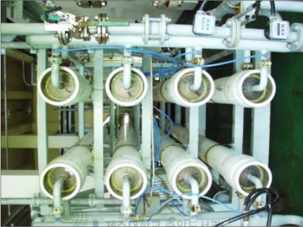
<Picture 2> RO Equipment Built in Udo Desalination Plant in Bukjeju County
