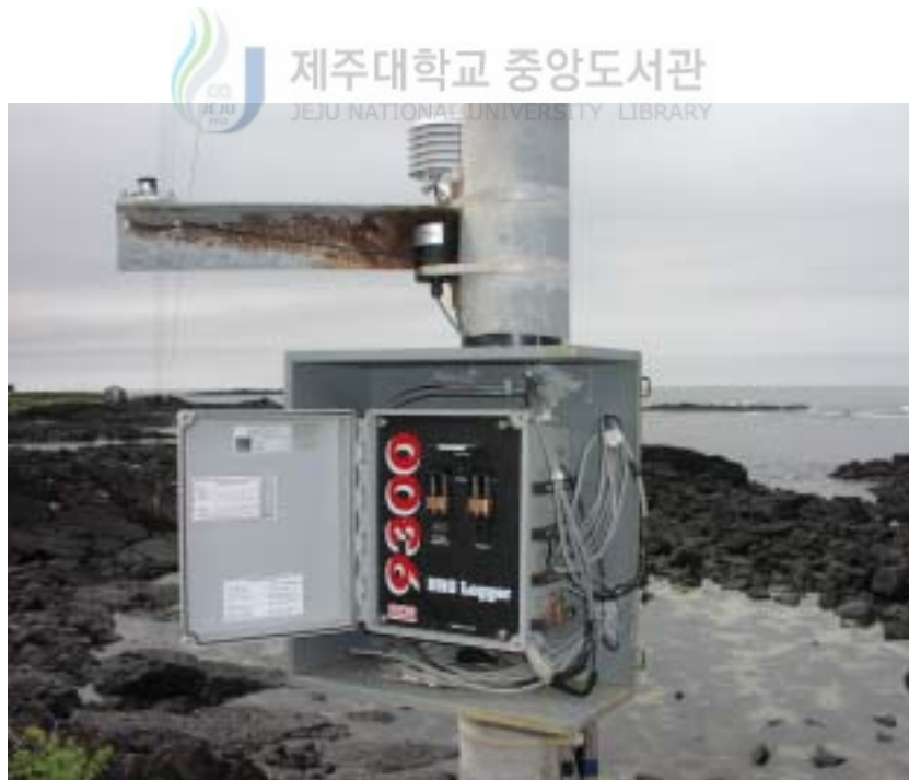
Fig. 17 The picture of data logger in Hangwon
