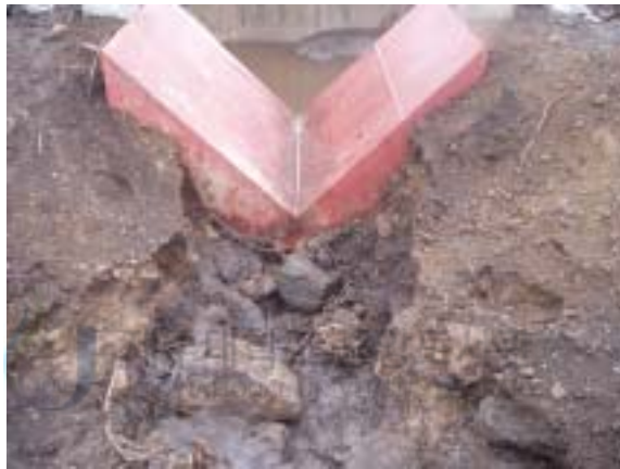
Fig 4.10 Photo of soil losse after rainfall
