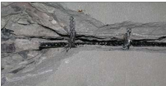
Fig. 4.12 CFRP grid tensile rupture(C4A-2T-1)
