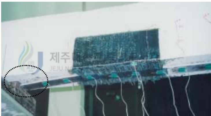
Fig. 5.7 Interfacial debonding failure(FP2)
