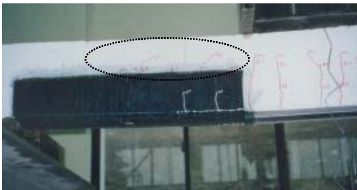
Fig. 5.8 Interfacial debonding failure(FP3)
